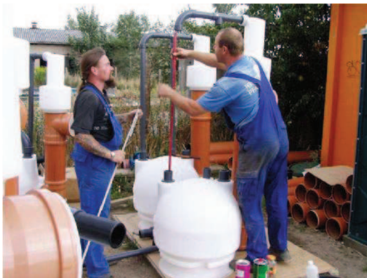
fig. 42 Measuring the pipe length of a G-Type collection chamber on building site
